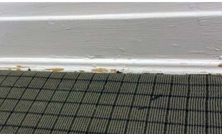
Baseboard paint can chip during the carpet installation
