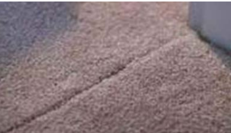
Unacceptable seam for plush carpet
