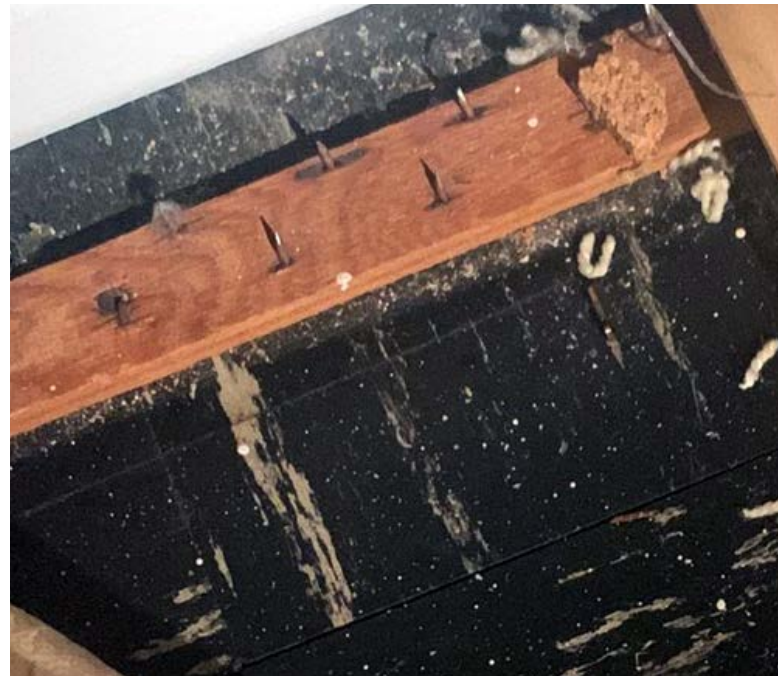
Typical asbestos tile
